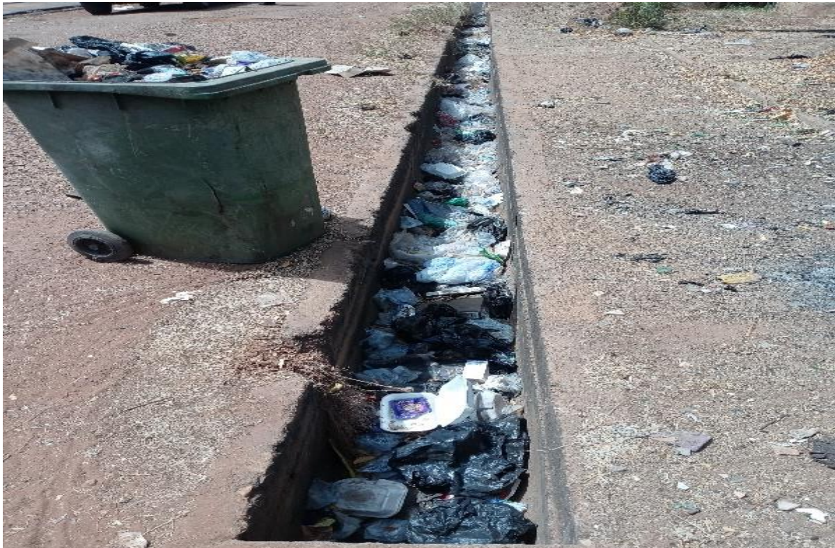
Picture 8: Open drain filled with plastics waste.
